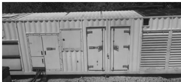
The new generator supplying 1.5 megawatts of electricity to Linden, Region Ten
