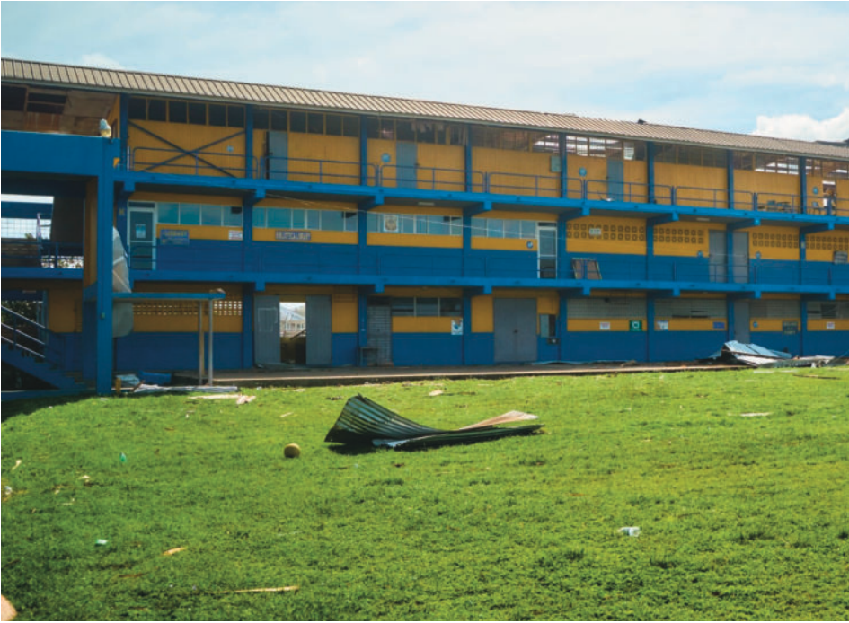
More than 300 schools were damaged by Hurricane Melissa
