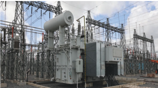
Infrastructure upgrades include new substations at Chateau Margot, Enmore, Columbia
