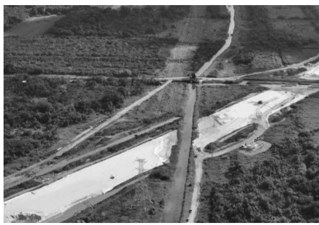
Aerial view of the construction works for the new Buzz Bee Dam to Land of Canaan four-lane highway
