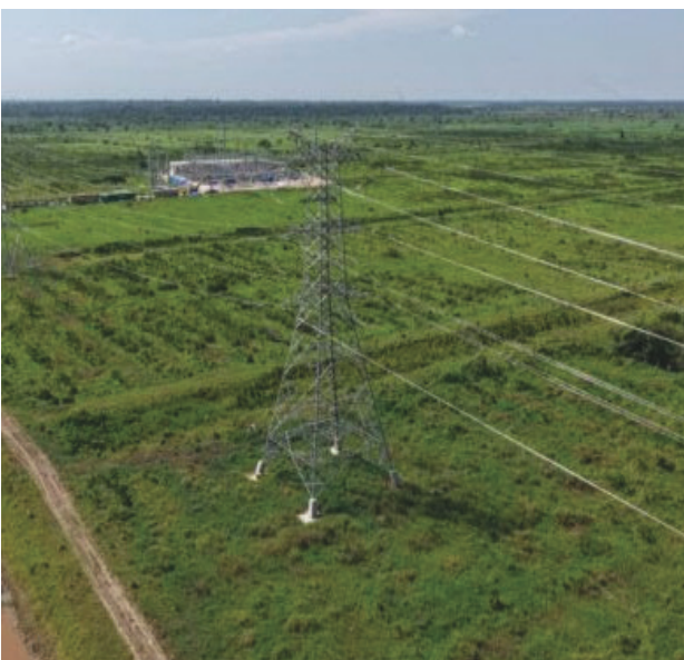
230Kv line tower with height ranging from 35-46 metres
