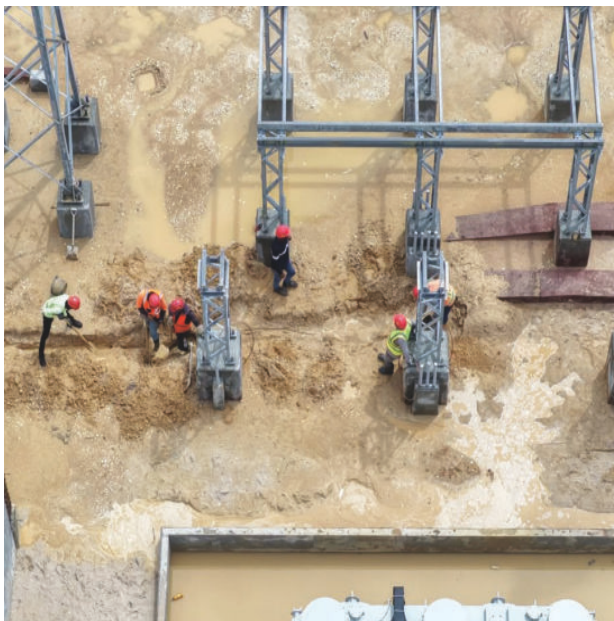
The Gas-to-Energy project remains a cornerstone of the Government's strategy to deliver reliable, affordable, and cleaner energy to Guyanese
