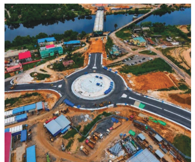
Roundabouts at both ends of the New Wismar-Mackenzie Bridge in Region Ten
