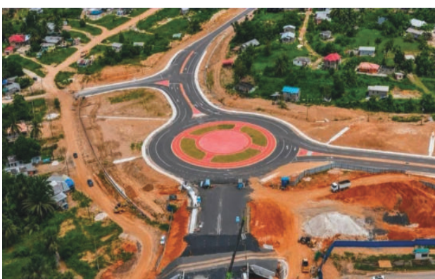
Roundabouts at both ends of the New Wismar-Mackenzie Bridge in Region Ten.
