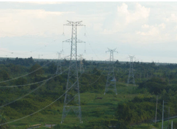
Electrical towers along the East Bank Demerara
