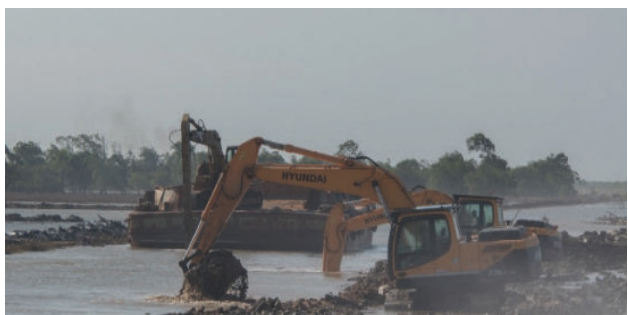
Excavators removing mud from Bellamy Canal to build a wall behind existing boulders along the foreshore in Mahaicony
