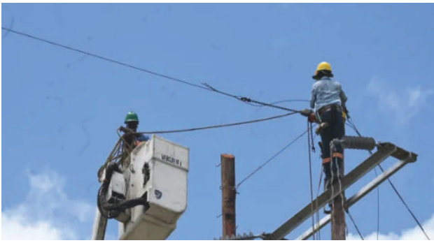
All utility lines will be removed as the 200-mile utility corridor is being built
