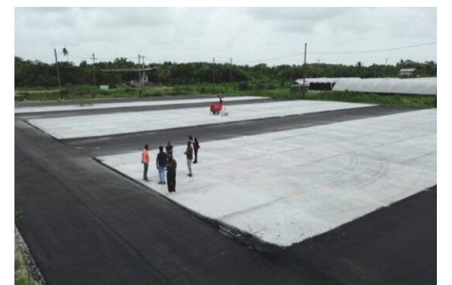
Minister within the Ministry of Public Works, Madanlall Ramraj, inspecting the new tarmac
