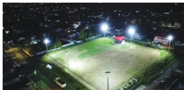
Lights installed at the Good Hope community ground
