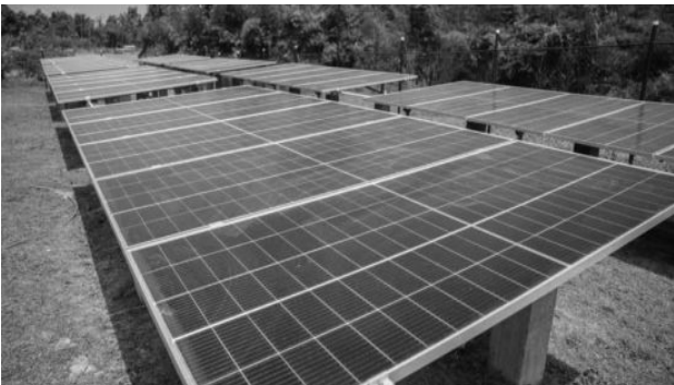
The commissioning of the solar grid
