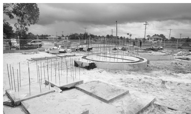
Five Miles water treatment plant
