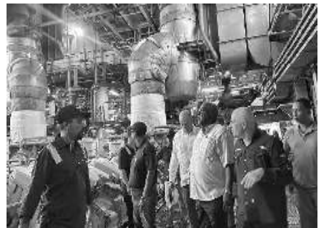
Prime Minister of Guyana, Brigadier R'td, Mark Phillips on a site visit to GPLs New Georgetown Substation and the Power Ship
