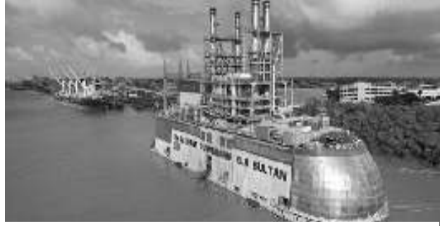
At approximately 1545 hrs on Monday, December 23, 2024, 60 Megawatts (MWs) of Generation was been added to the grid.
