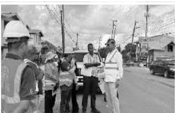
Minister of Public Works, Bishop Juan Edghill conducting an inspection of the works being done on the Ogle to Eccles Road Project
