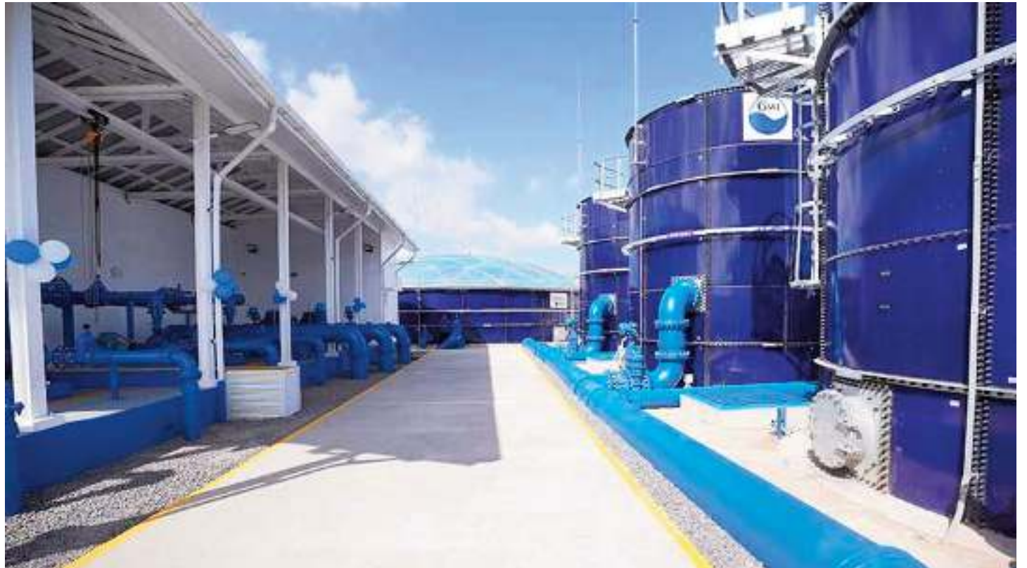
One of the new water facilities
