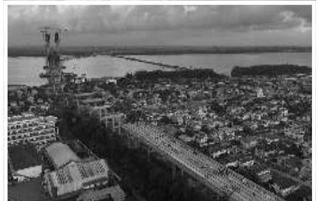
An overhead view of works on the US$260 million new Demerara Harbour Bridge
