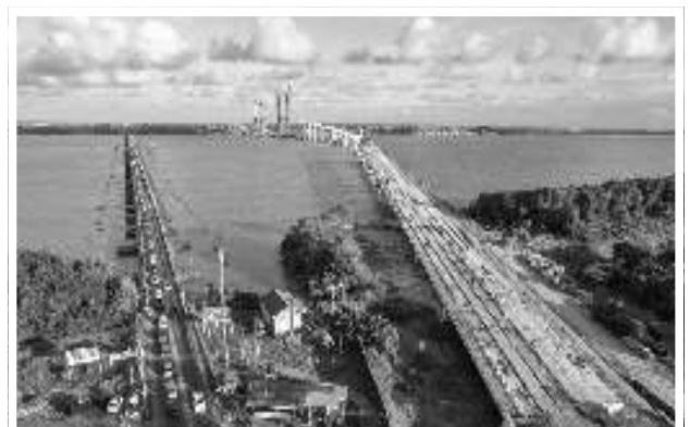
Construction of the new Demerara River Bridge rapidly progressing (Things Guyana image)
