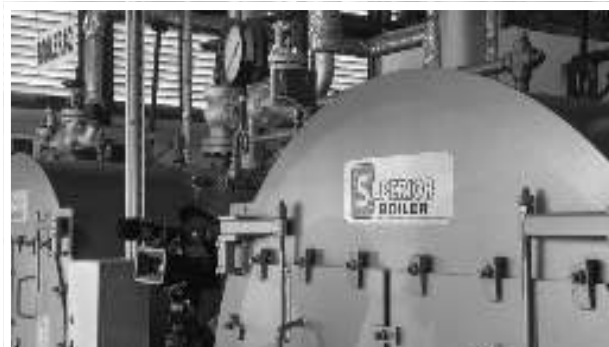
The new boiler
