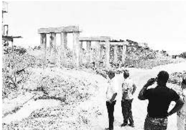
Minister of Public Works, Bishop Juan Edghill, engineering team and contractor inspecting works on the Pirara bridge
