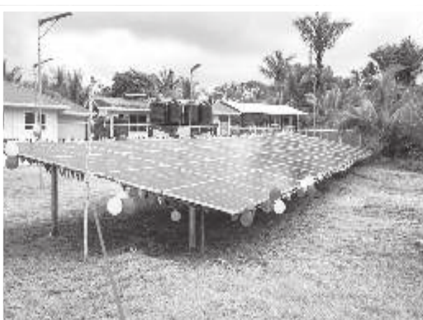
One of the two, solar PV systems
