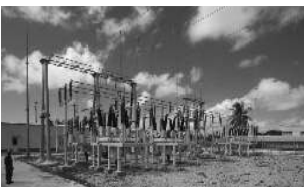
A $160 million investment will upgrade GPL's transmission and distribution system
