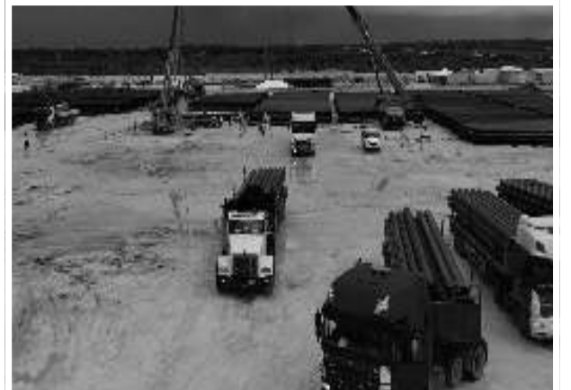
The project development at Wales on the west bank of the Demerara River
