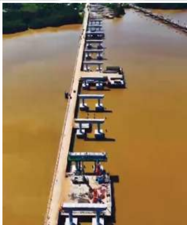
The construction of the new Demerara River Bridge and its connecting infrastructure
