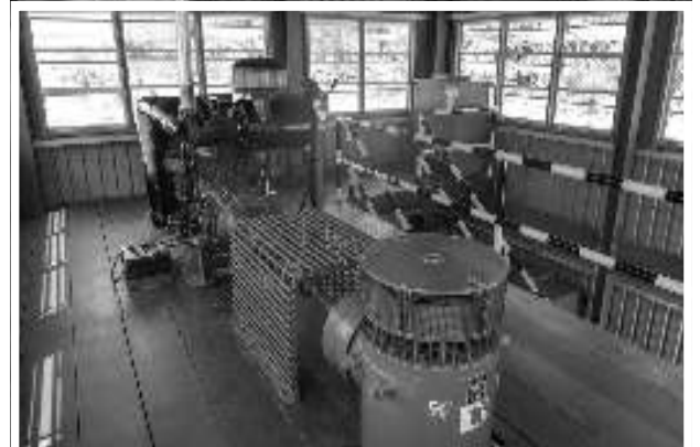
Inside the pump station
