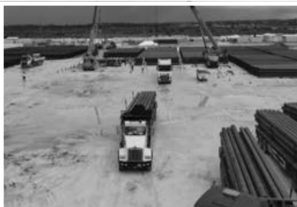
The multi-billion-dollar gas to energy power plant, which is currently under construction at Wales, West Bank Demerara
