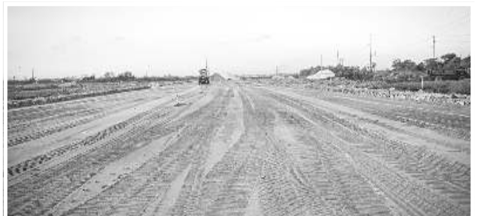
Ongoing works on the four-lane road from Diamond to Buzz Bee Dam (Craig)
