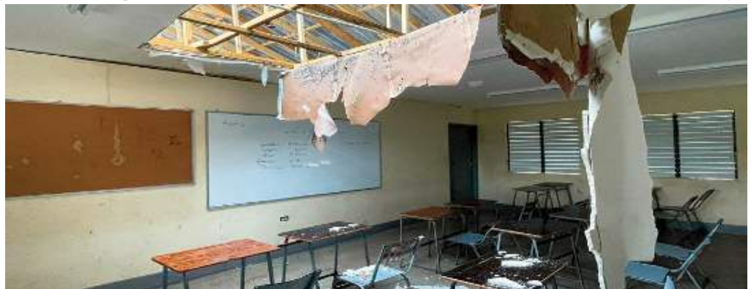
A school in Jamaica damaged by Hurricane Beryl
