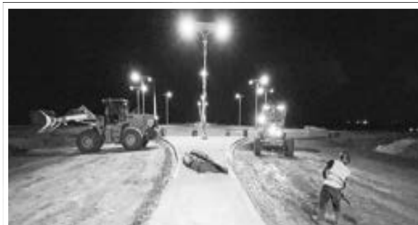
Working the night shift to complete the Schoonord to Crane four-lane highway by the end of the month
