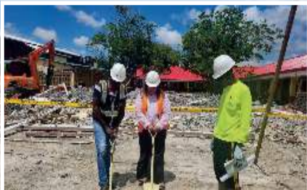
Sod turning for the construction of a brand new wing at Tucville Secondary School
