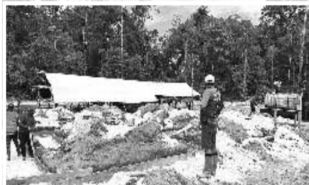
Ongoing works at 5 Miles Housing Scheme Phase II in Bartica, Region Seven
