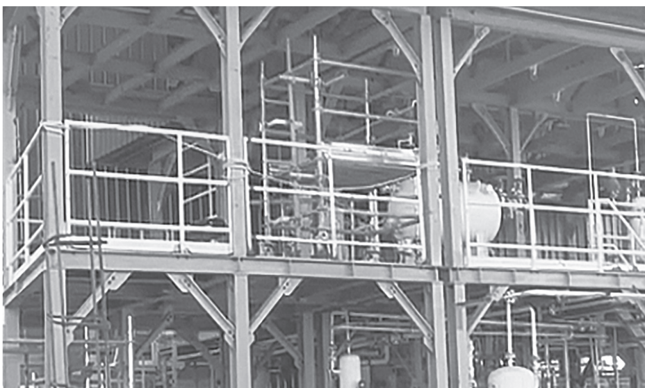
Construction progressing on the Port Mourant National Oil and Gas Training Centre
