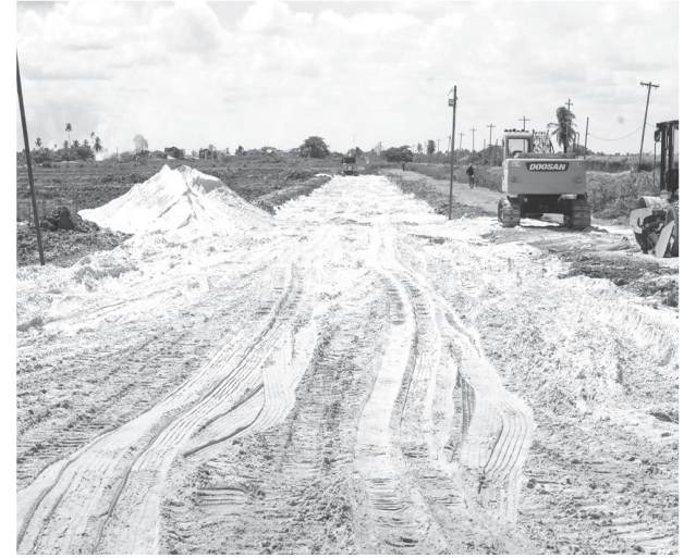
Construction of a road that will service the development of the community
