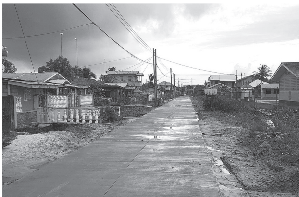
One of the newly constructed roads in the Parfaite Harmonie Housing Scheme
