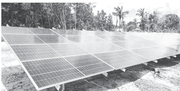
The solar farm in Mission Capoey boasts a 41.5-kilowatt system; while Tapakuma's solar mini-PV farm provides residents with a 21-kilowatt system
