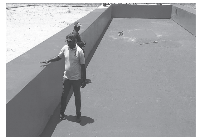
The 25 m X 20 m pool which took approximately over a month to be constructed
